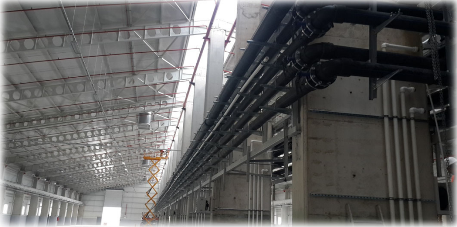
Mutlu Battery, Process Piping System
