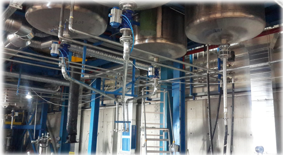
Server Boya Food Coloring Production Boilers
