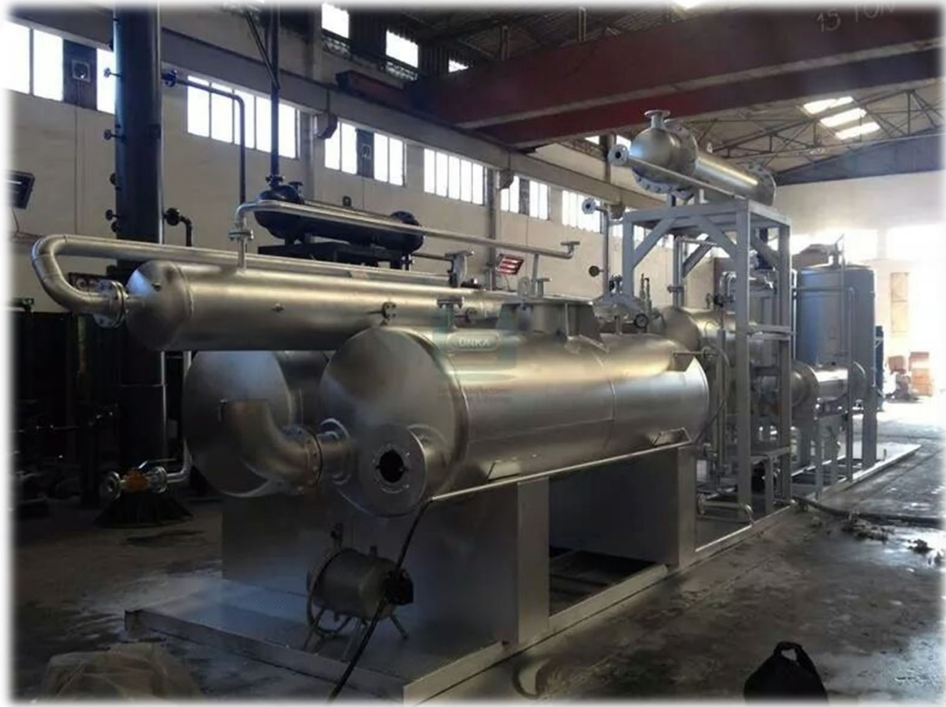
Process Piping and Alternative Fuel Equipment
